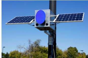
Figure 1. Autonomous, solar-powered device with computer controlled color mirror mounted on utility pole.
